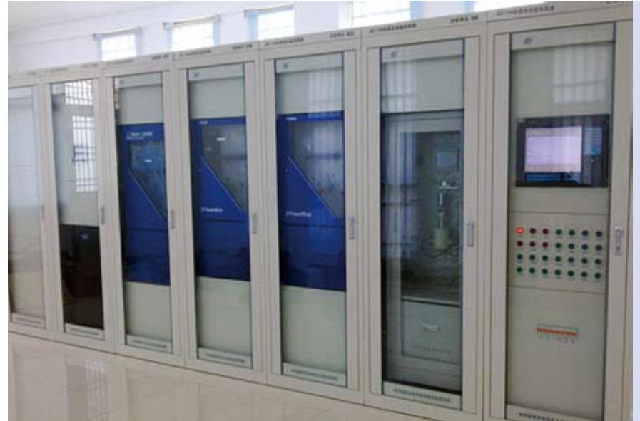
• 武进港水质站 Water quality station, Wujin port
